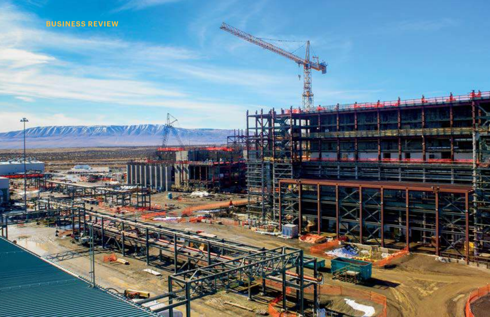
▲ Hanford Waste Treatment and Immobilization Plant Washington, USA
