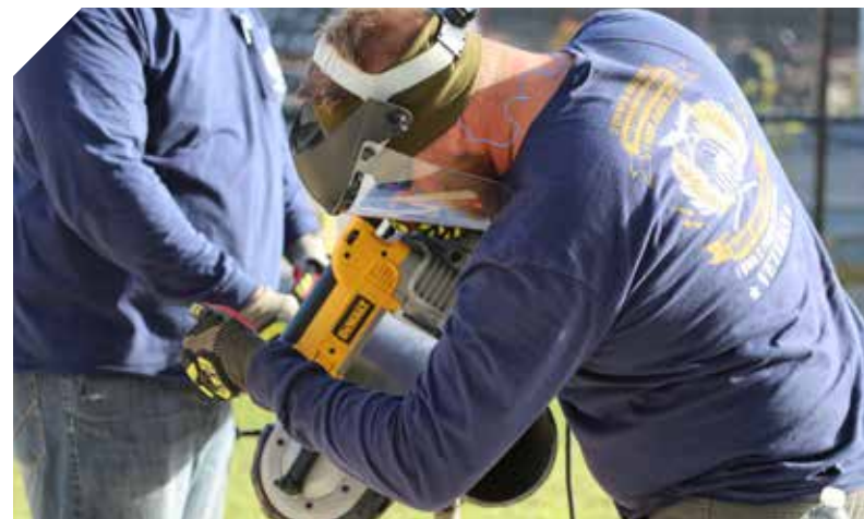
Student demonstrates the proper technical cutting of pipe and proper use of bandsaw during his class at the Bechtel Welding and Applied Technology Center.
