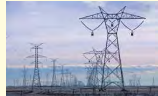
Eastern Alberta Transmission Line, Alberta
