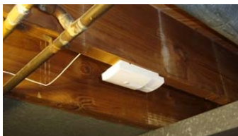
CO MONITOR INSTALLED NEAR HEATING SYSTEM
