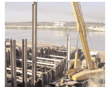
Installing H-pile for retaining wall of a power plant in central Iraq where Bechtel built new generation units
