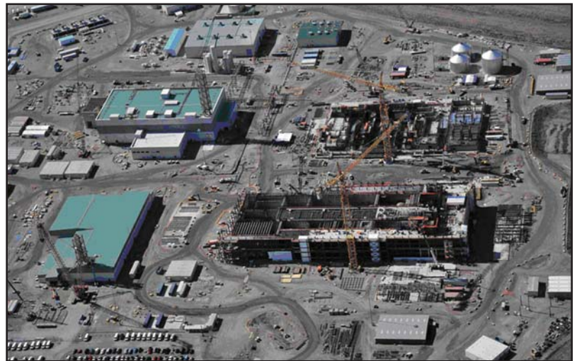
Figure 1. Hanford Waste Treatment Plant Facilities, Washington State
