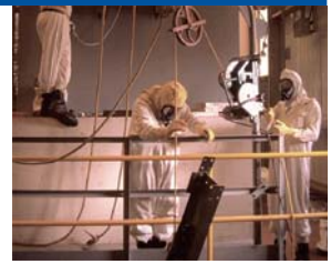
Once inside the containment building, engineers and technicians installed television cameras to monitor the cleanup.
