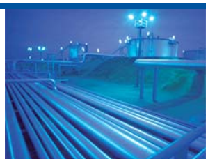
Bechtel was central to the full restoration of oil production and refining in Kuwait.
