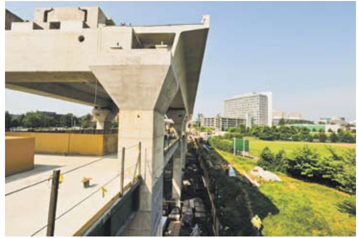
The first phase of the Metrorail extension to Dulles International Airport and Loudoun County has thus far provided contracts to 171 local small businesses owned by ethnic minorities and women, creating hundreds of jobs. File photos by Joanne S. Lawton
