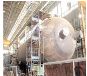
Palo Verde 2 - The largest steam generators in the world
