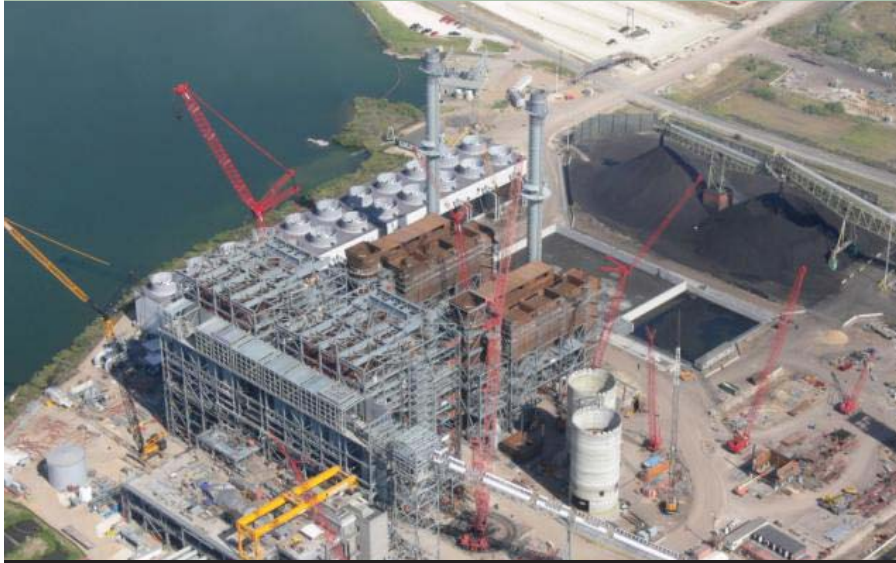
The Sandow Steam Electric Station Unit 5 is being built adjacent to existing units.
