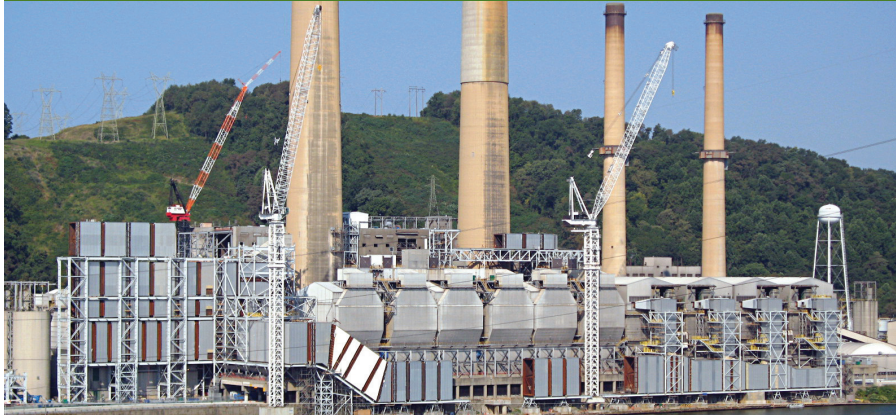
Sammis Retrofit Project—installing air quality control systems on seven units, totaling 2,200 MW
