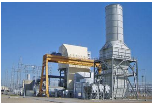
Completed Kirkuk v94 Power Plant
