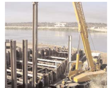
Installing H-pile for retaining wall of a power plant in central Iraq where Bechtel is building new generation units
