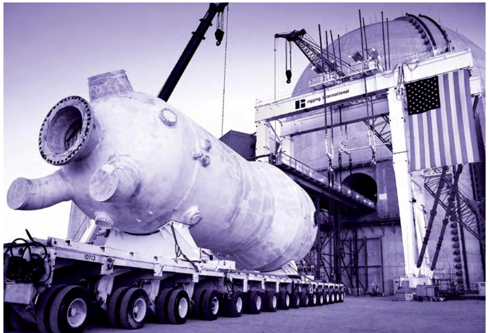
A steam generator is removed at Palo Verde Nuclear Generating Station in Arizona.
