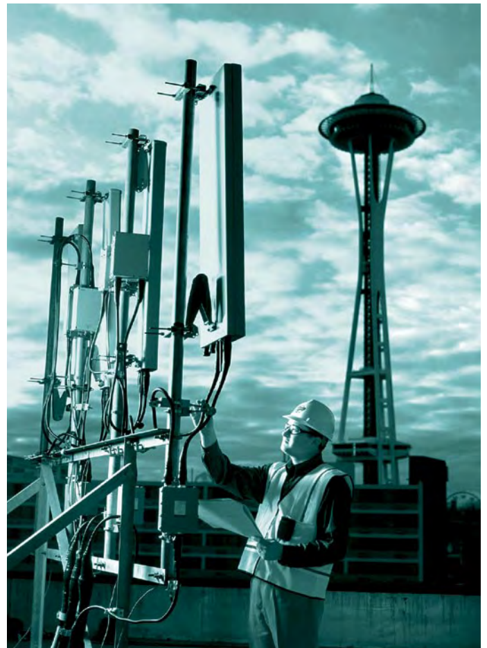
Antennas of a Cingular rooftop cell site in Seattle, Washington.
