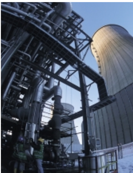
Power plant program, Turkey
