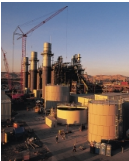
Delta Energy Center, California
