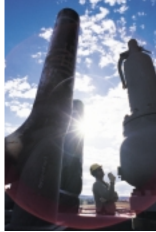
Nearing completion ahead of guaranteed schedule, the Millmerran power facility southwest of Brisbane is Queensland’s first fully privatized power project.
