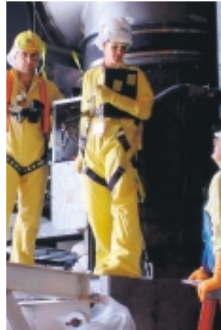
Replacing two steam generators at Wisconsin's Kewaunee nuclear power plant, Bechtel helped return the facility to full operation in just 71 days.
