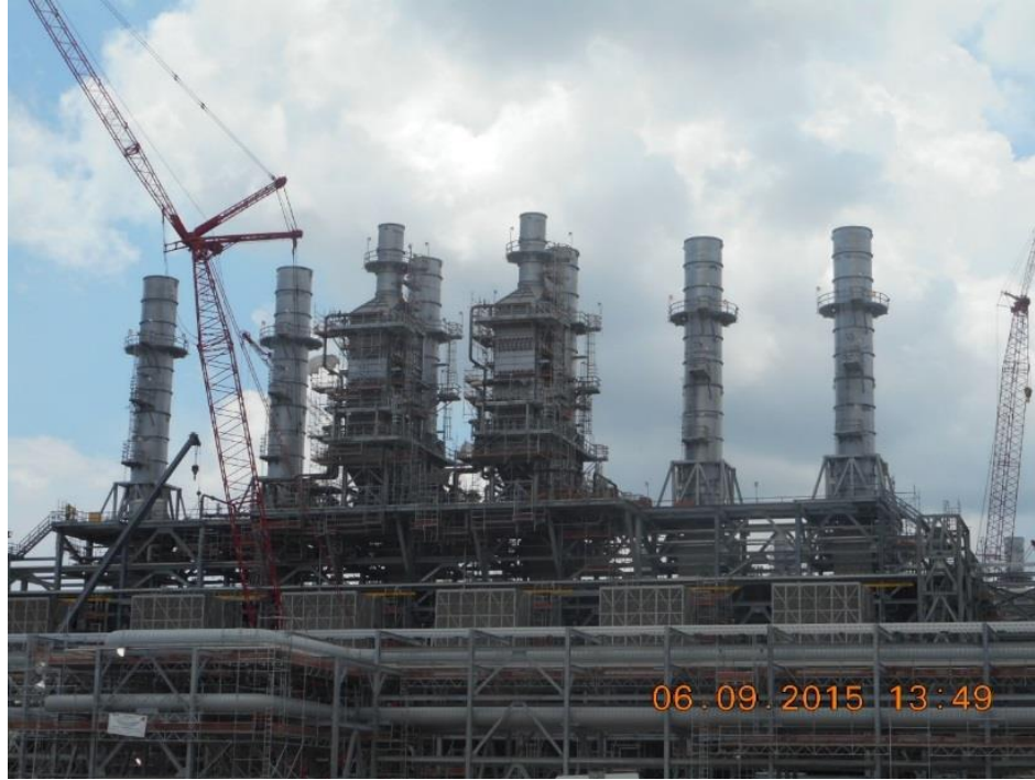
Figure 15 - Waste Heat Recovery on Ethylene Gas Turbine Exhausts
