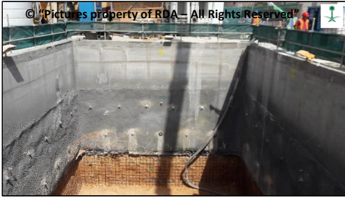
Figure 6. Excavation in deep alluvium supported by a combination of retaining wall and nailing.
