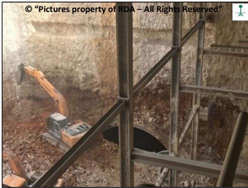
Figure 11. Large infilled cavity exposing alluvial/aeolian soil above tunnel crown in station excavation.
