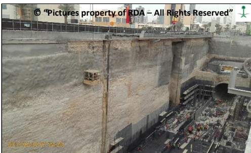
Figure 7. Combination of retaining wall and nailing for soil support above vertical excavation in massive breccia.
