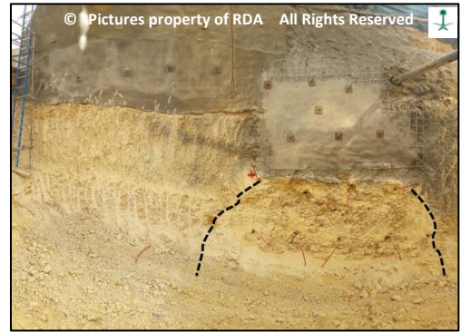
Figure 10. Stabilization of infilled cavity.
