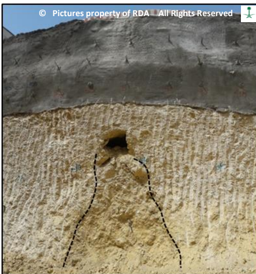
Figure 9. Infilled cavity exposing collapsed material.
