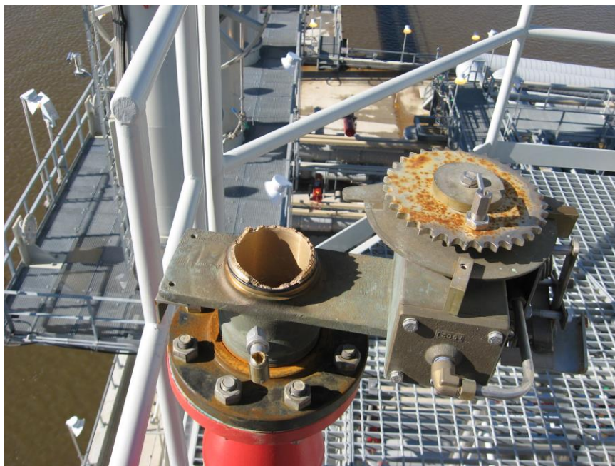
Figure 2 Result of dry pipe start-up test
